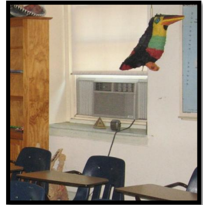
Image 9-Window AC unit used as means for air conditioning,
